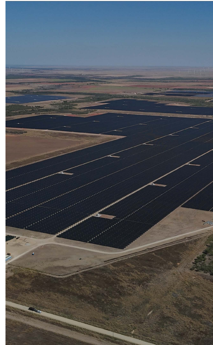
The Millers Branch Solar Facility in Haskell County, Texas (pictured right) is expected to come online in 2026.
